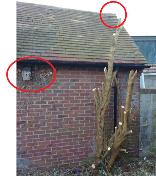
Photograph 12 Western elevation visible after buddleia shrubs had been removed, with bird nesting box attached to building, and slipped and lifted tiles visible on roof covering.
