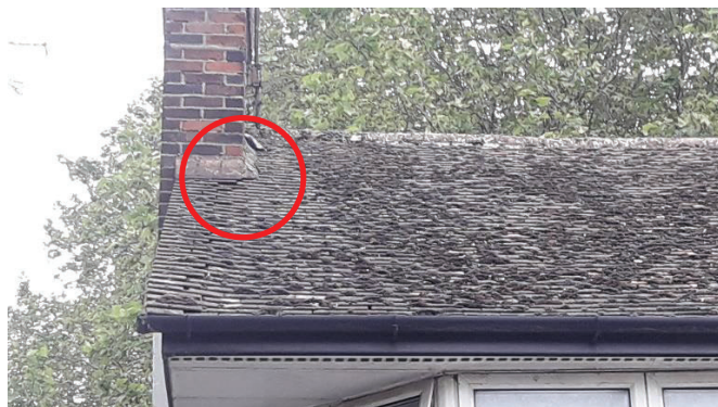
Photograph 4 Example of gap under roof tile on Building B11, to the south of the chimney.
