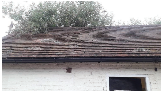
Photograph 10 South-eastern elevation of building B16, with several lifted/slipped tiles on the roof covering.
