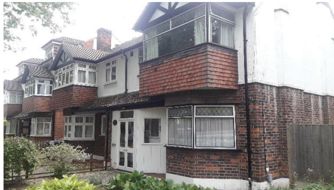
Photograph 3 View of B11, as viewed from the north-west on Kingfield Road. Representative view of hanging tiles beneath bay windows.
