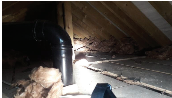
Photograph 2 View of inside of loft void of Building B10, appears to have been recently re-roofed with breathable membrane lining the tiles.
